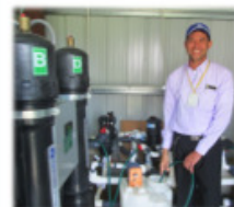
Hospital staff preparing chlorine solution next to GE ultrafiltration system, La Esperanza
